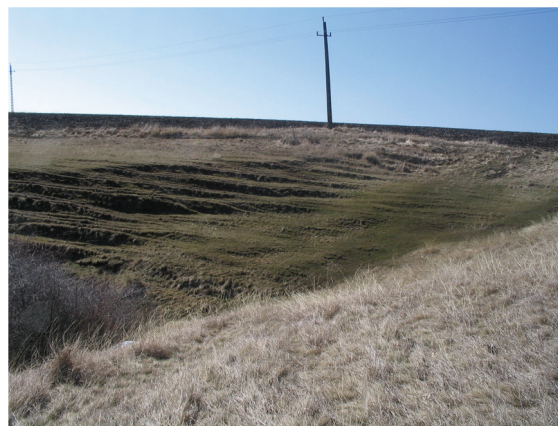
Fig. 12. Landslides in Bogács
